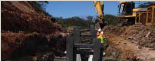
$16 million invested at the Caloundra Landfill to minimise site impacts on the water quality of Lamerough Creek.
